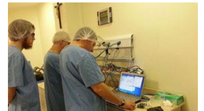
Figure 4: HSVP surgical room with Protegedem installed inside the gas and electric outlets panels. The figure shows the installation moment in which the calibration for the correct measurement of the leakage current values is made.
